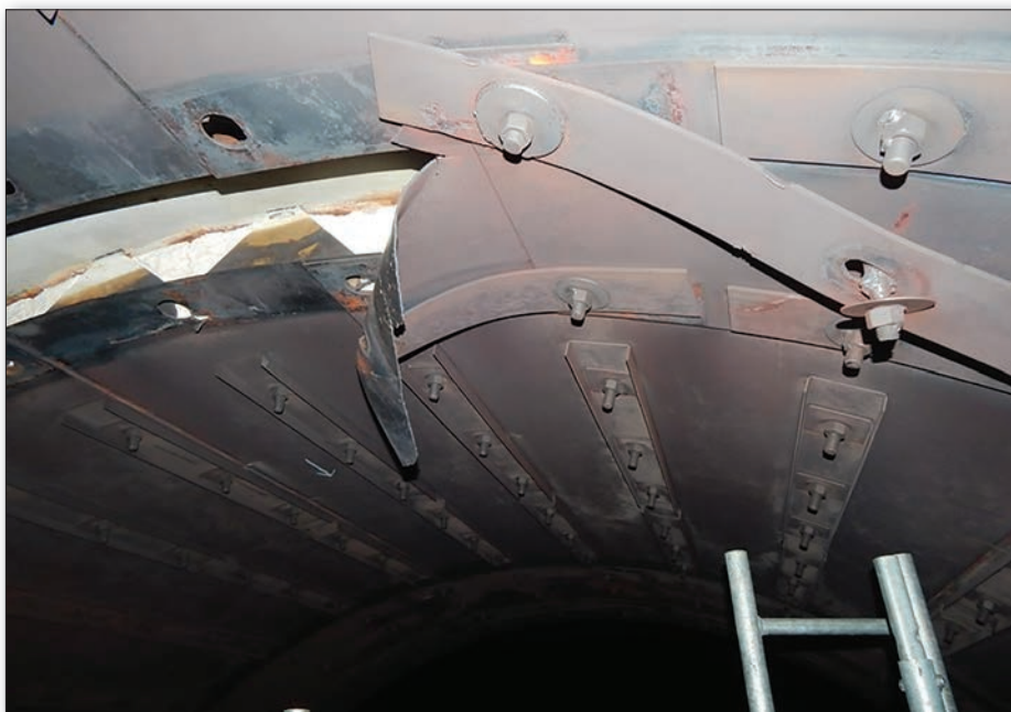
Figure 2: As fired hours and starts accumulate, so do the chances of finding broken studs in this section
