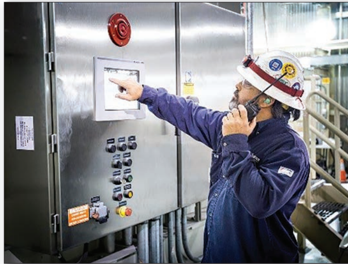
An operator at a Solar Turbines control panel
