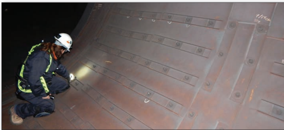
Figure 1: F-class turbines often have a round diffuser duct between the gas turbine and the downstream HRSG or stack
