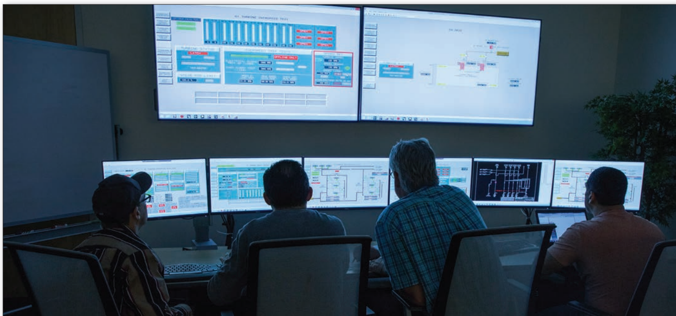
Emerson Automation Ovation controls monitor turbomachinery and plant assets
