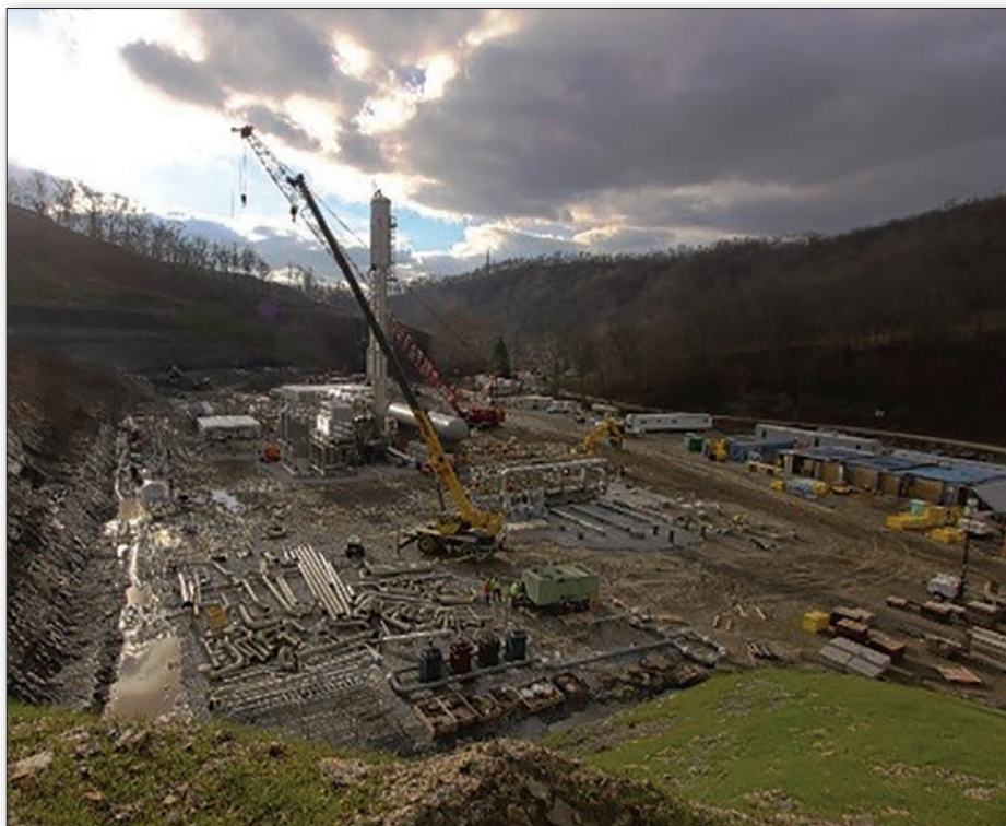
UOP Russell Modular Gas Plant
