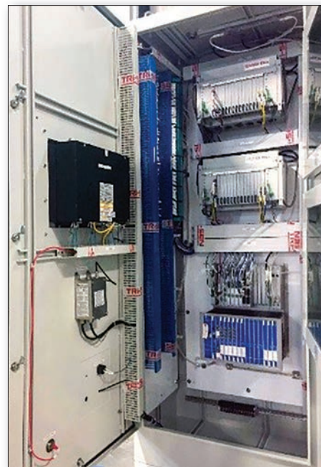
Redundant Tri-Sen TSx system for a steam turbine-driven Elliott recycle compressor at a plant in Egypt
