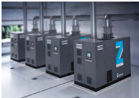
Atlas Copco variable speed drive centrifugal blowers
