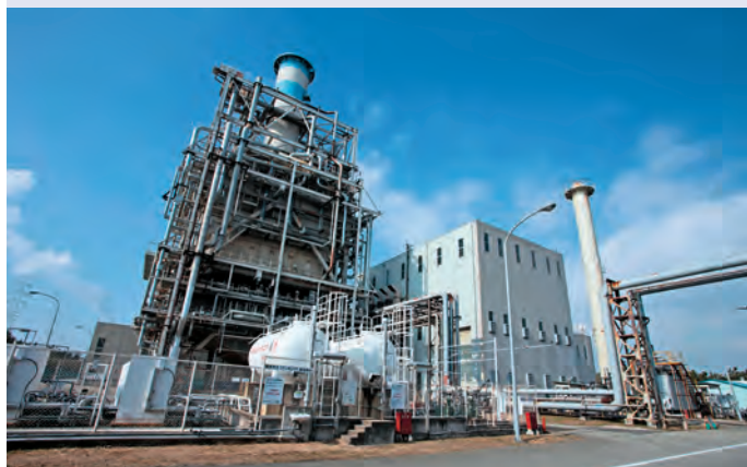
The MHPS T-point gas turbine combined cycle demonstration facility in Japan is being used to develop a machine capable of running at firing temperatures of 1,700°C.
